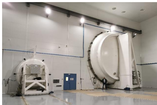
Both TVAC installed in the clean room
