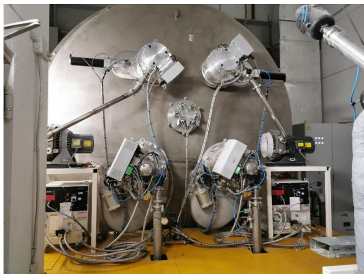
High Vacuum Pumping System
