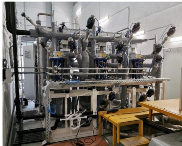
Thermal System with 2+1(spare) lines
